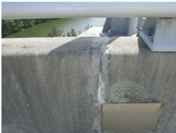
S3 방호벽 균열( C_w=0.2/L=0.6m )
