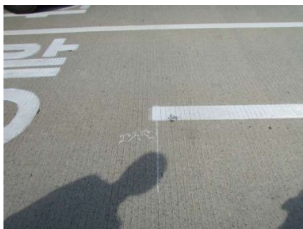
S3 LMC포장균열( C_w=0.5/L=3.0m )
