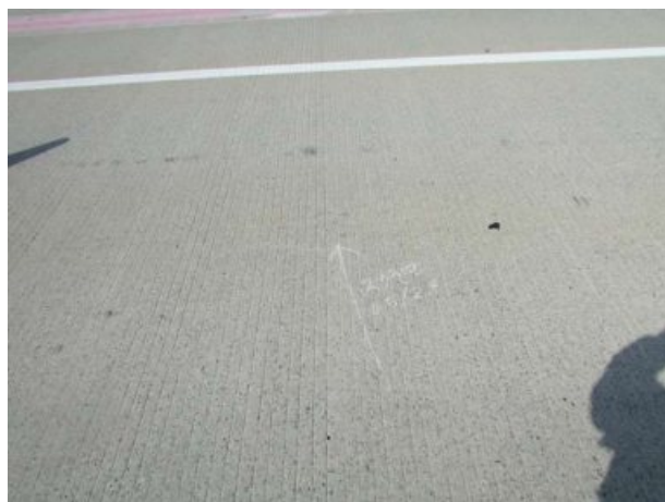
S2 LMC포장균열( C_w=0.5/L=2.0m )
