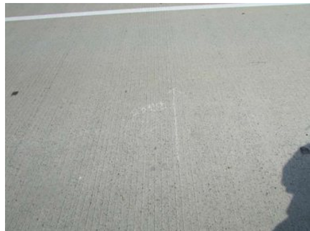
S3 LMC포장균열( C_w=0.5/L=2.5m )
