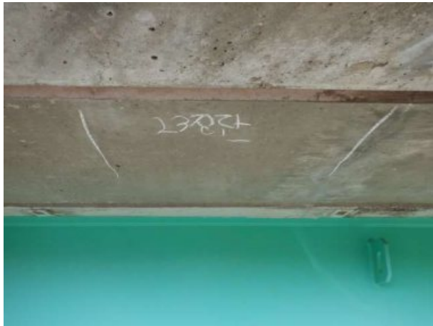
S2 캔틸레버 균열( C_w=0.2/L=0.6m )
