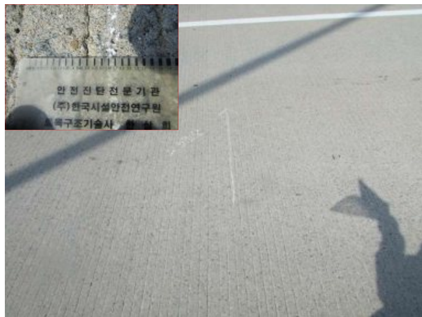
S3 LMC포장균열( C_w=0.5/L=3.5m )
