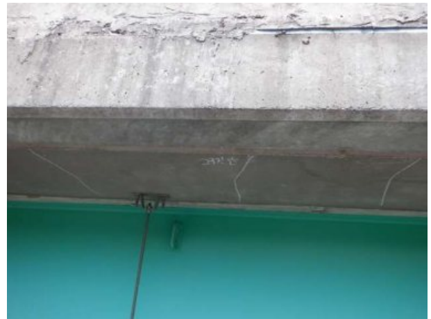
S4 캔틸레버 균열( C_w=0.2/L=0.6m )
