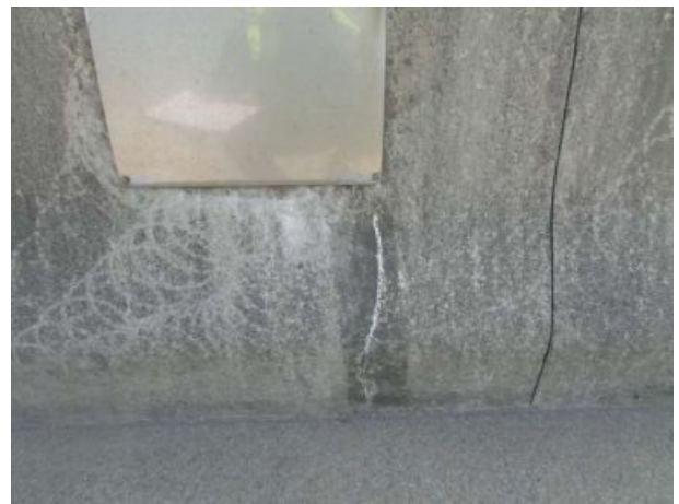
S3 방호벽 균열( C_w=0.2/L=0.4m )
