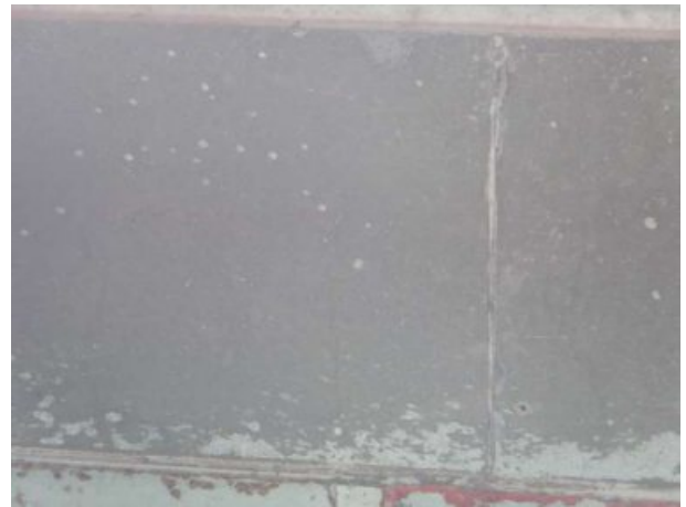
S3 캔틸레버 균열( C_w=0.2/L=0.6m )
