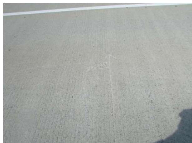
S3 LMC포장균열( C_w=0.5/L=2.5m )
