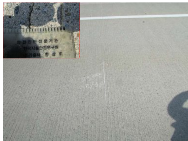
S2 LMC포장균열( C_w=0.5/L=3.0m )
