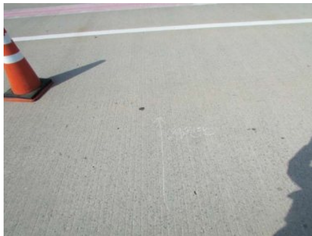
S4 LMC포장균열( C_w=0.5/L=3.0m )
