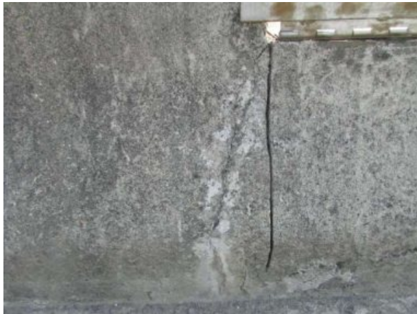
S3 방호벽 균열( C_w=0.2/L=0.5m )
